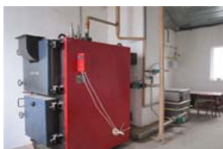
Industrial hot water boiler purchased with funding through an AgroInvest grant
